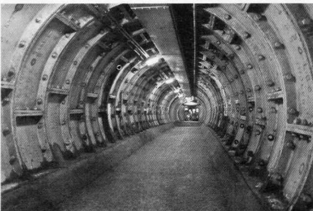
This section of the Woolwich foot tunnel was repaired during WWII. Photo Mike Peel
